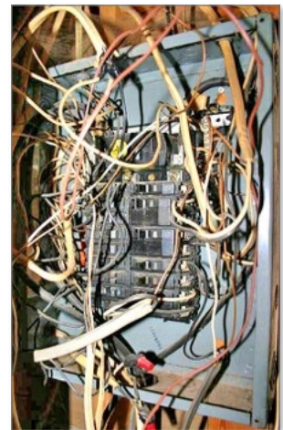
example: Electrical Code violation
