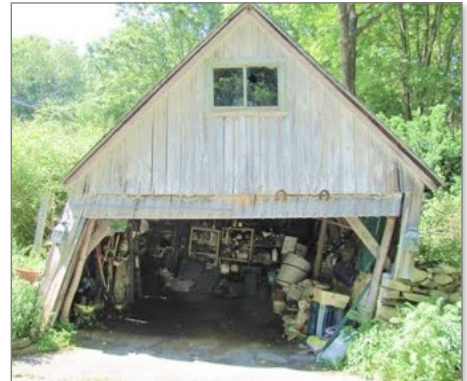
example: Dangerous / Unsightly Structure
