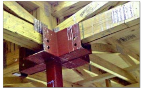
example: Building Code violation
